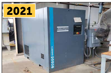
60HP Atlas-Copco Air Compressor
