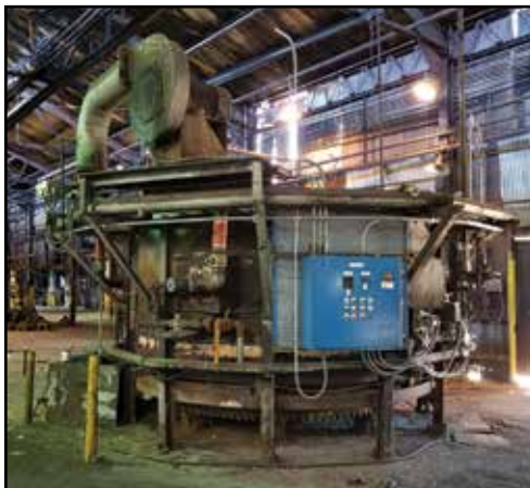
(16) Gas Fired Slot, Hearth & Fire Box Furnaces
