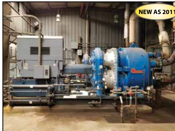
(2) INGERSOLL RAND Centac 2,250-HP Centrifugal Air Compressors
