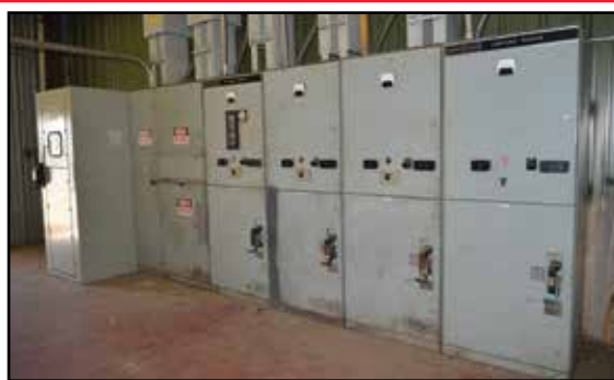
GENERAL ELECTRIC 7700 Line Motor Control Center
