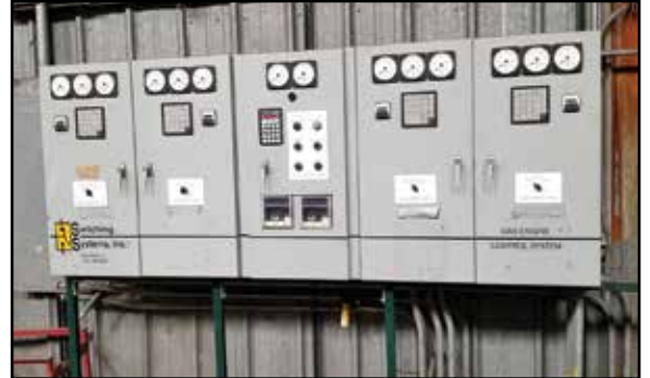
5-Panel Switching Systems Gas Engine Control System
