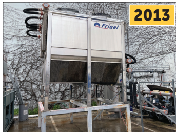
Frigel Chiller and Tower
