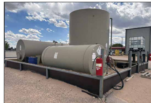
Fuel Depot to Include: 2013 Edge 5,000 Liter Horizontal Off-Road Diesel Tank, Etc.
