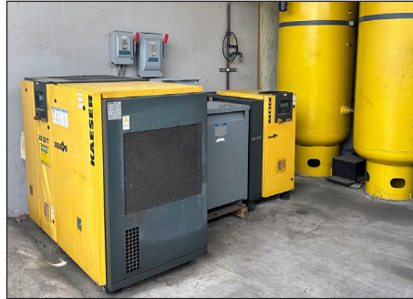
Kaeser Air Compressor
