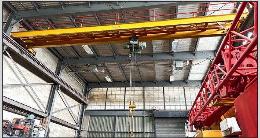
7.5-TON BRIDGE CRANE
